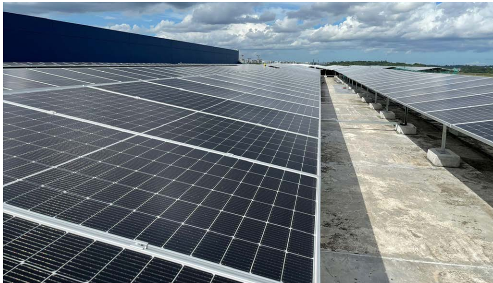
> Solar panels at Regional eCommerce Logistics Hub (LogHub)
